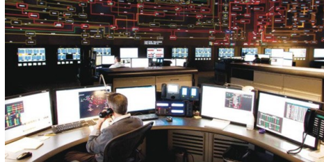
NYISO control room | NYISO
